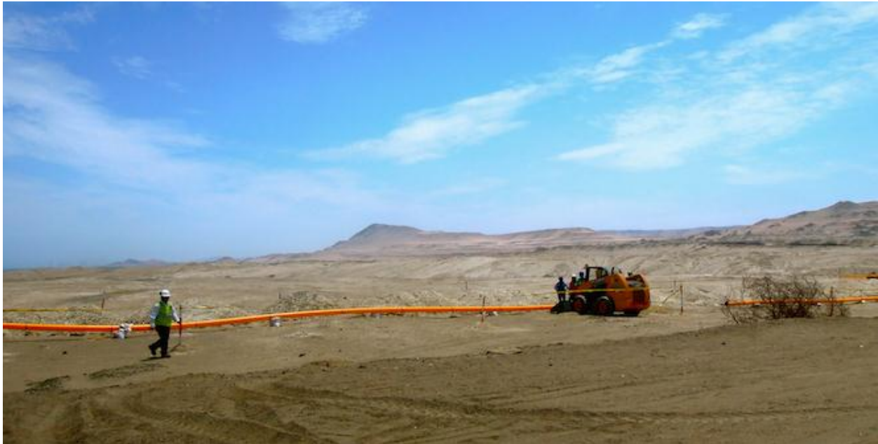
Construction work on natural gas pipelines in the Marcona desert Photo credit: Caitlin Duffy
